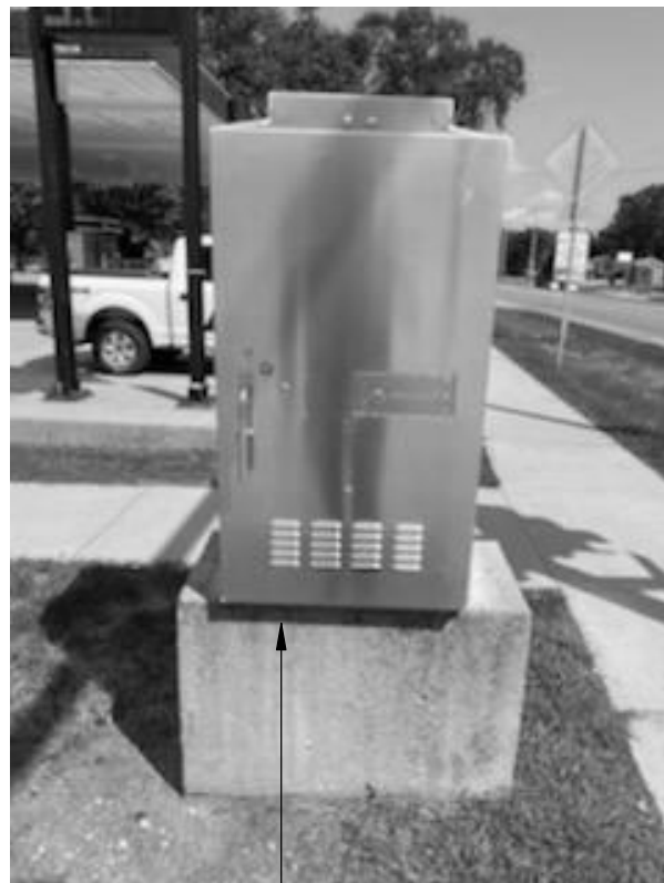
ENCLOSURE EXAMPLE OF NEW EQUIPMENT AT 3RD AND MAIN STREET
